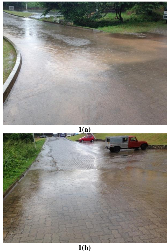
Figure 1: Water pooling in front of Faculty of Engineering due to a small rainfall
